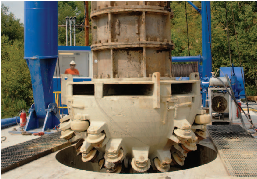
The reamer body for the shaft drilling system is lowered into the hole.
